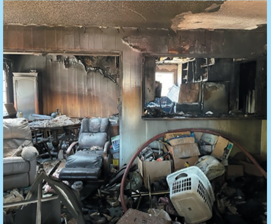
On July 21, at 8:45 am, the Ventura City Fire received a call of a reported structure fire in the 400 block of Nova Court. Upon arrival firefighters found a well involved single family residence with a report of a person trapped inside. Firefighting crews immediately entered the building fighting fire and conducting a search for a victim. A deceased female was located inside the home. Firefighters extinguished the fire 14 minutes after arrival. One adult male was treated and transported to the hospital for burns and smoke inhalation sustained while attempting to extinguish the fire with a garden hose.
