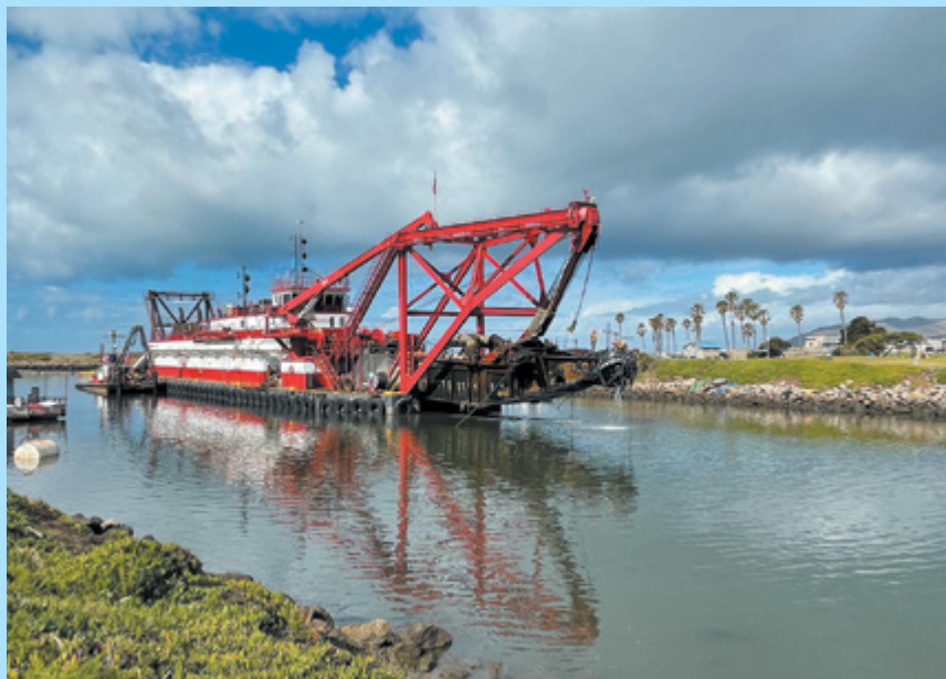
An estimated 485,000 cubic yards of material has been removed from the entrance channel and placed upon the beaches.
