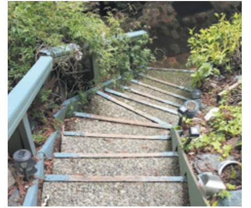
Uneven stairs can result in dangerous falls.
