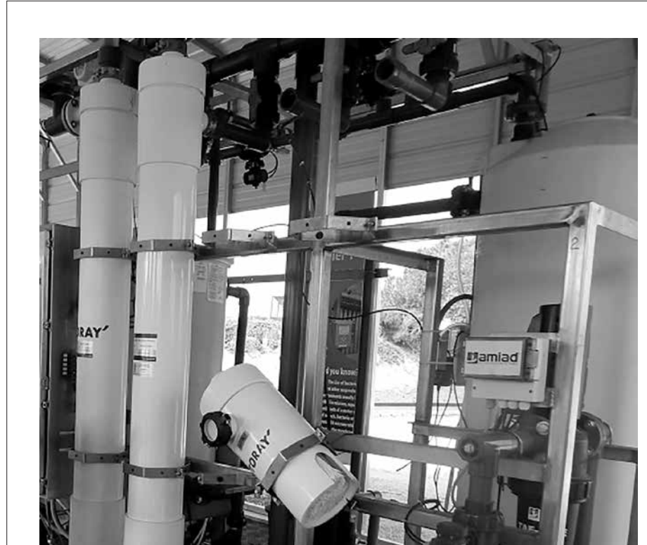
Congresswoman Julia Brownley (CA-26) and Ventura Mayor Cheryl Heitmann will tour the VenturaWaterPure Demonstration Facility (located at 1400 Spinnaker Dr.-Ventura Water Reclamation Facility) on Thursday, October 15. Ventura Water, in partnership with the Water Research Foundation, is utilizing the demonstration facility to; generate essential research, better inform regulators on how to move from indirect potable reuse to potable reuse blending, and to help create a secure water future for the City of Ventura. Congresswoman Brownley says, "I look forward to visiting the VenturaWaterPure Potable Reuse Facility, and learning more about how this facility will meet the needs of local water users. As we look for solutions to the drought, California must embrace innovative ideas, like water reuse and recycling, which are playing an increasing role in meeting our unprecedented water challenges."
