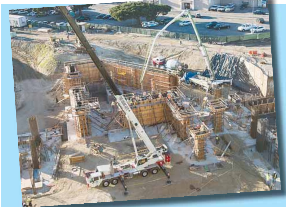
The first wall of the new Community Memorial Hospital has been poured.
