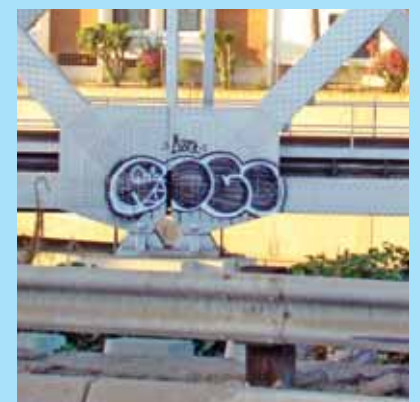
Even though the railroad trestle is still looking great where there is a will there is a way as the first major graffiti has been applied to the trestle. If you ever see graffiti being applied to any surface by these criminals please immediately call 911.
